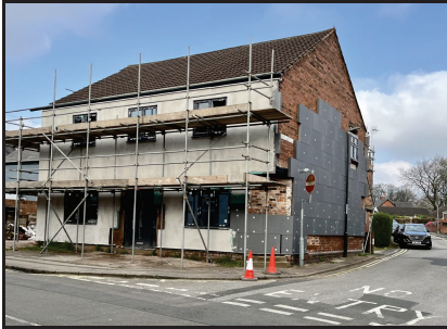
A house on Calow Lane on which external cavity wall insulation is currently being fitted.
